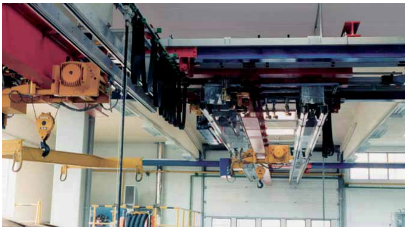
Aluminium enclosed conductor system on crane bridge.
