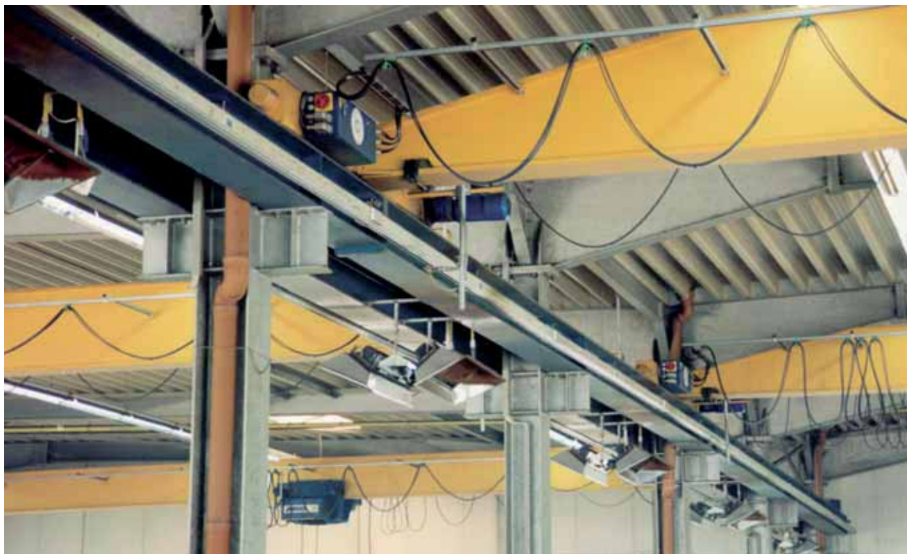
Aluminium enclosed conductor system for crane electrifications.
